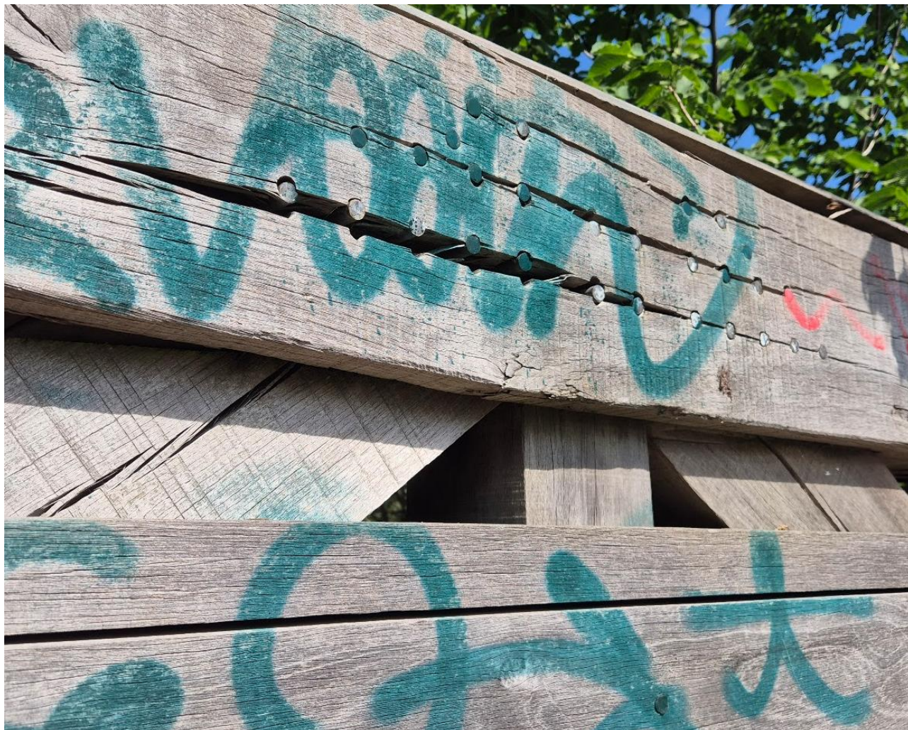
Figure 1: Top chord node – severe splitting in all members. Note right-hand diagonal displacing up and left-hand diagonal pulling down
